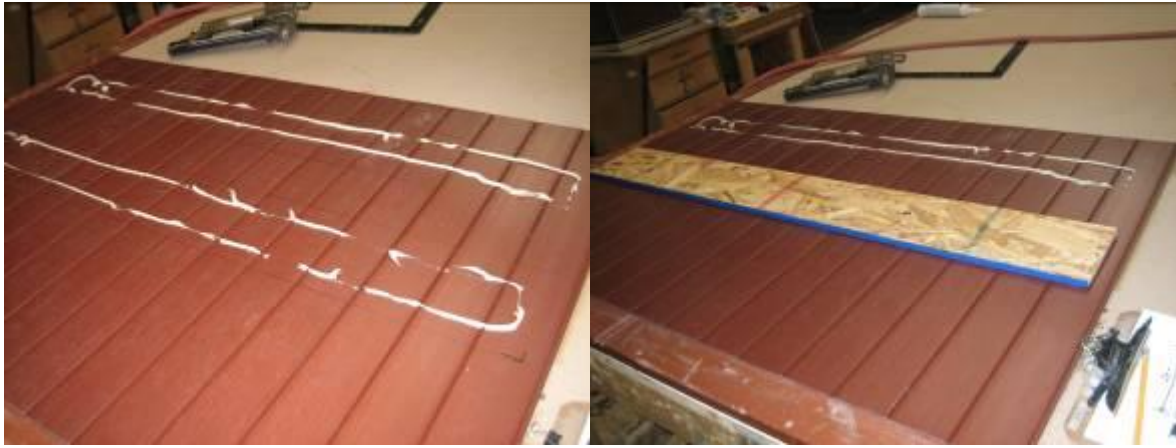
Images 7&8: Beads of adhesive in backer location & backing boards pressed in place
